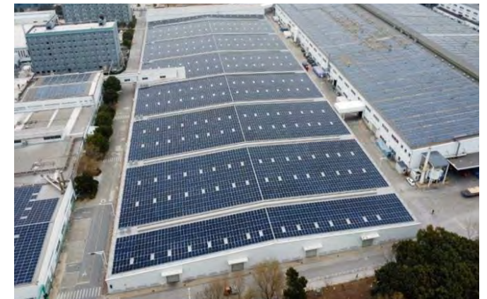
Rooftop Photovoltaics at the Hisense Huzhou Air Conditioner Factory
